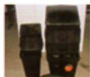
Distribution & Drop Boxes
